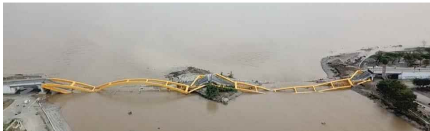
Figure 7.4 Palu IV Bridge Was Collapsed
