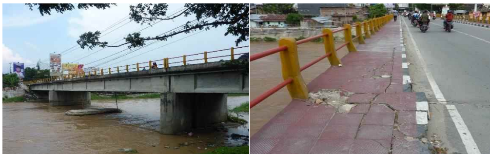
Figure 7.5 Superstructure of Palu I Bridge was Moved to 20 cm
