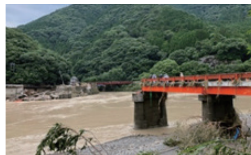
Kuma River, Collapsed Fukami Bridge (Yatsushiro, Kumamoto Pref.)
