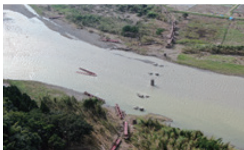
Kuma River, Collapsed Kuma River Bridge No. 4 (Sagara-Nishiki-cho, Kuma-gun, Kumamoto Pref.)
