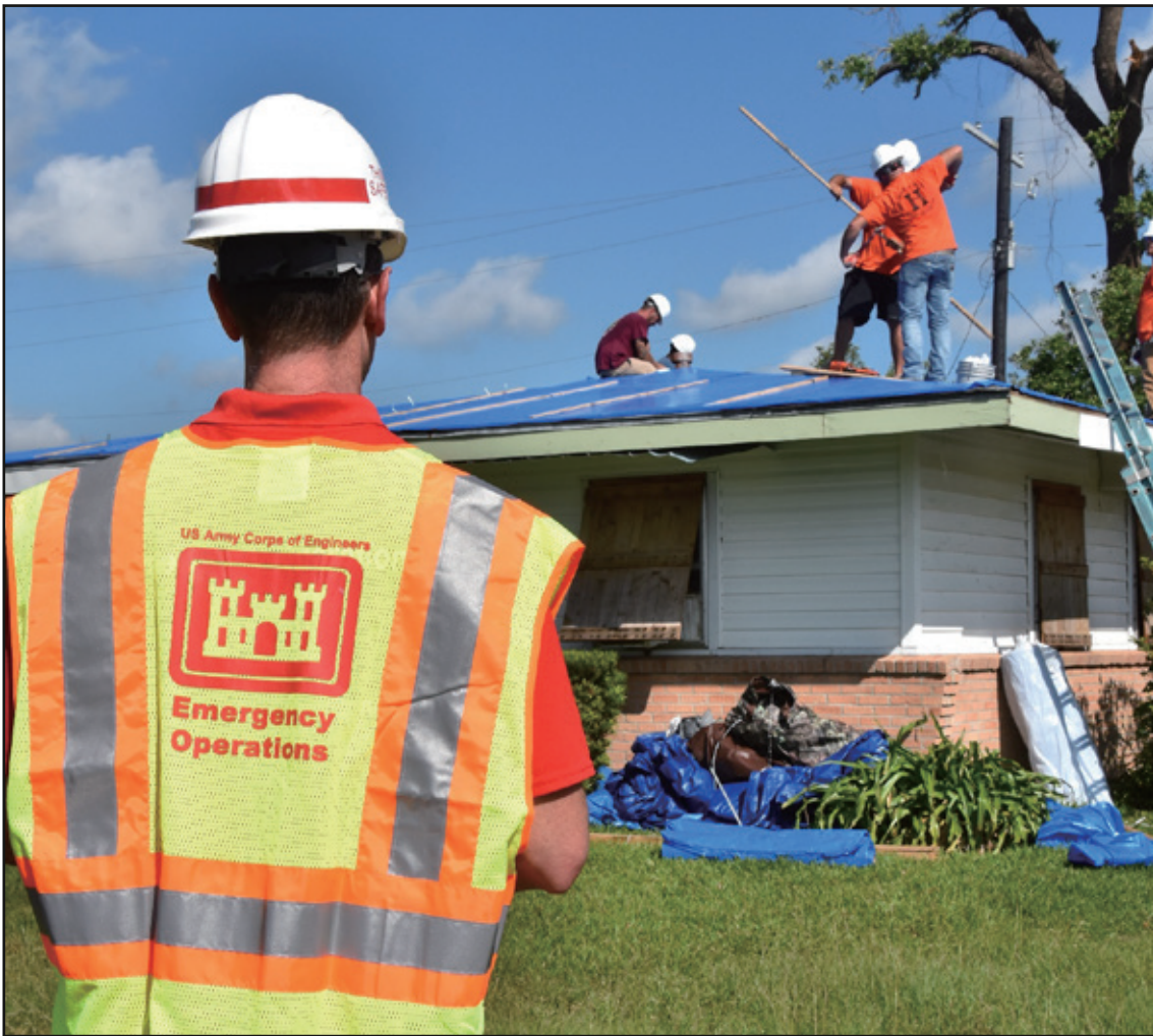
Figure 7. A U.S. Army Corps of Engineers' Blue Roof Mission Assessor observes contractors as they install temporary roofing for the 5,000th homeowner to receive a 'blue roof' during Hurricane Laura recovery efforts. Using satellite and fixed-wing imagery allow USACE assessors anywhere in the world to conduct assessments, but if for some reason imagery is unclear, an evaluator will conduct a physical review of the roof to ensure an accurate assessment is conducted. (Photo by George Stringham, USACE St. Paul District)
