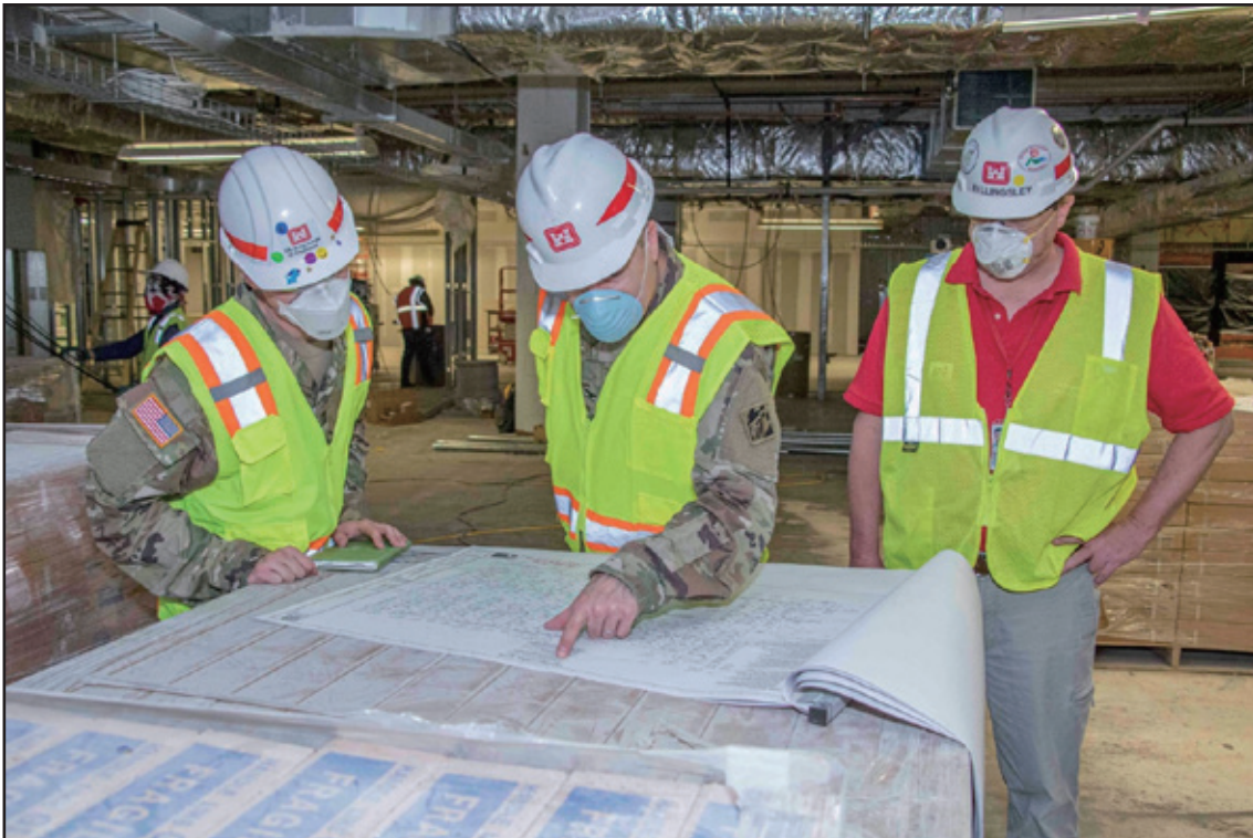
Figure 1. USACE Memphis District Commander Col. Zachary Miller visited the former Commercial Appeal building April 29, 2020, for a progress update tour of what became Memphis' only USACE-built Alternate Care Facility. (USACE photo by Vance Harris)
