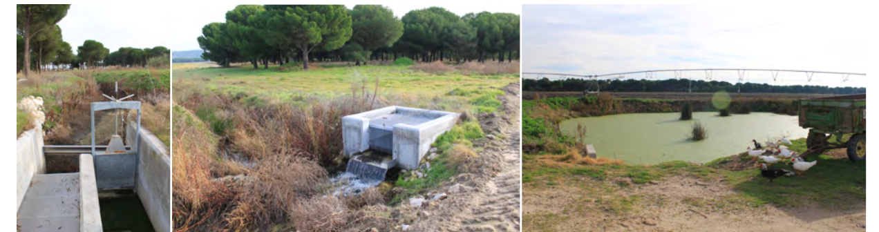
The Pedrajas-Alcazarén MAR scheme: (a) connection point where the flows from the WWTP, rooftop runoff and Pirón River diversion converge; (b) valve where the pipeline feeds the infiltration canal; and (c) previous sandpit reused as infiltration pond (source: TRAGSA).
