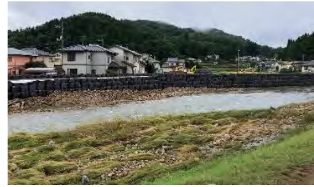
Levee Broken (Tajihigawa River)
